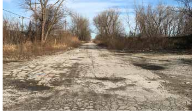
Poor pavement conditions on Stony Island Avenue between 122nd Street and the Calumet River/Lake Calumet in the City of Chicago.
