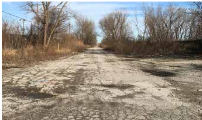
Poor pavement conditions on Stony Island Avenue between 122nd Street and the Calumet River/Lake Calumet in the City of Chicago.
