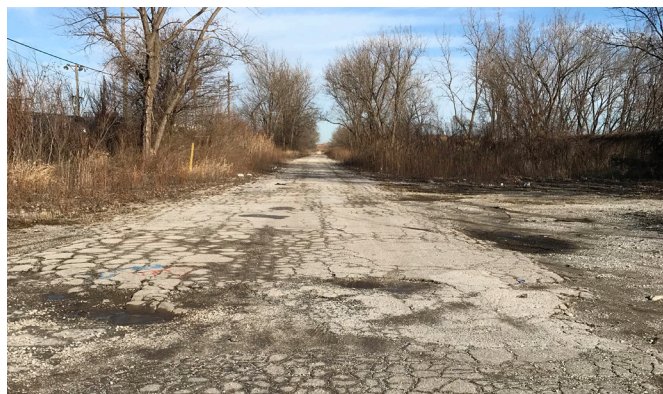
Poor pavement conditions on Stony Island Avenue between 122nd Street and the Calumet River/Lake Calumet in the City of Chicago.
